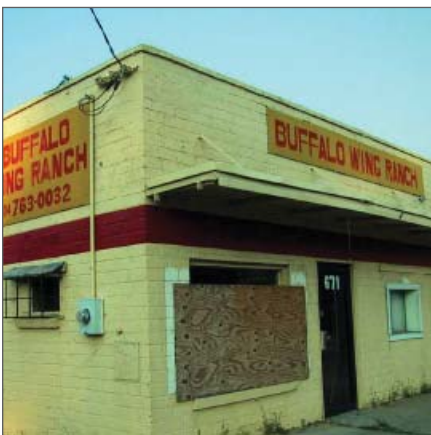
Dilapidated storefront on North Central Avenue before rehab (Hapeville). Average score: - 4.1
